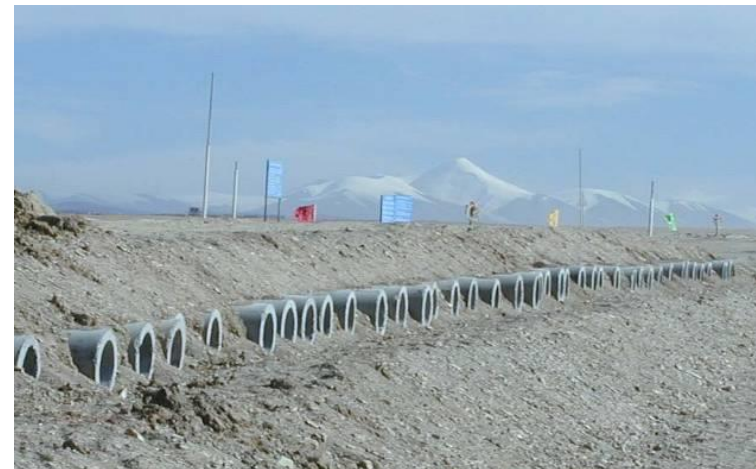
Pipeline ventilation roadbed of Qinghai-Tibet railway
